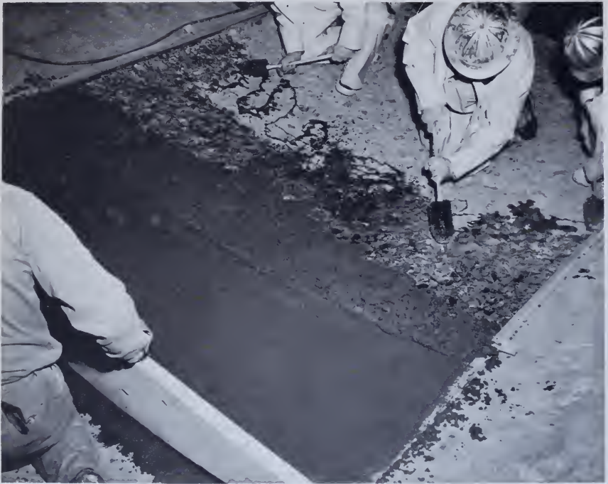
Figure 183. —Epoxy bond-coat being applied to prepared concrete surface before placement of new concrete. New low-slump concrete must be placed while the epoxy bond-coat remains fluid. P622A-427-15035.
